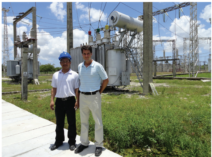
MDU retrofit by Huaming in Cuba in 2006. Since then it has been working properly.
